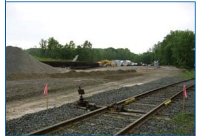
All States Asphalt's new site at E. Deerfield, MA with track panels stacked, waiting for installation Photo Credit: Mike Clements
